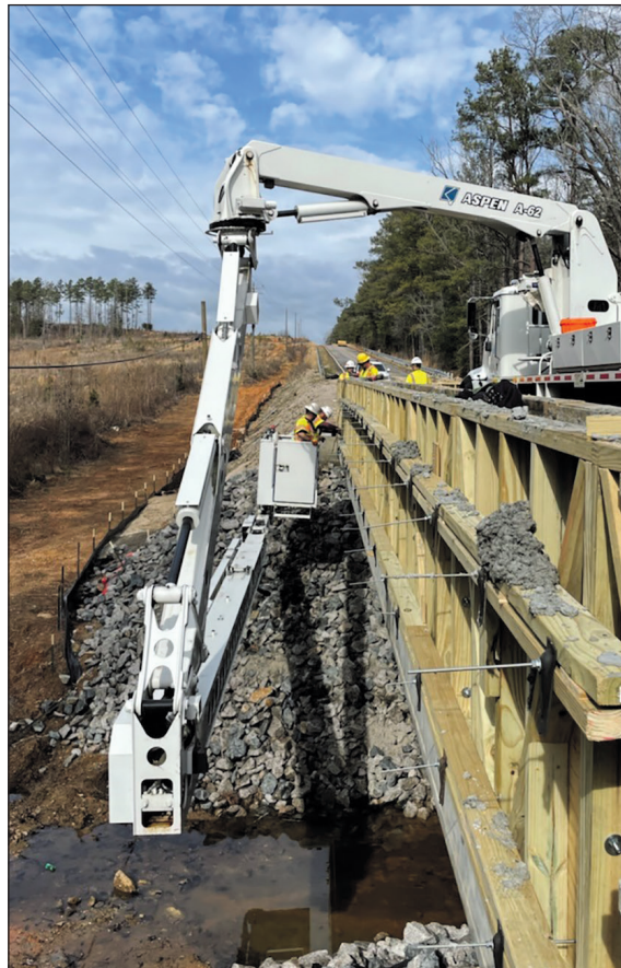
Harold Ballard and Jesse Jordan work on the outside of the wall forms while Branden Bozard controls the bucket. This bridge is S.C. 97 over Rocky Branch Creek in Kershaw County.
