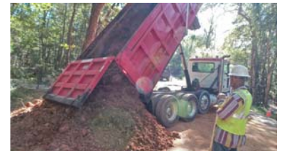
Contractors from Taylor Brothers, a certified minority contractor, make repairs along Congress Road in lower Richland County.
