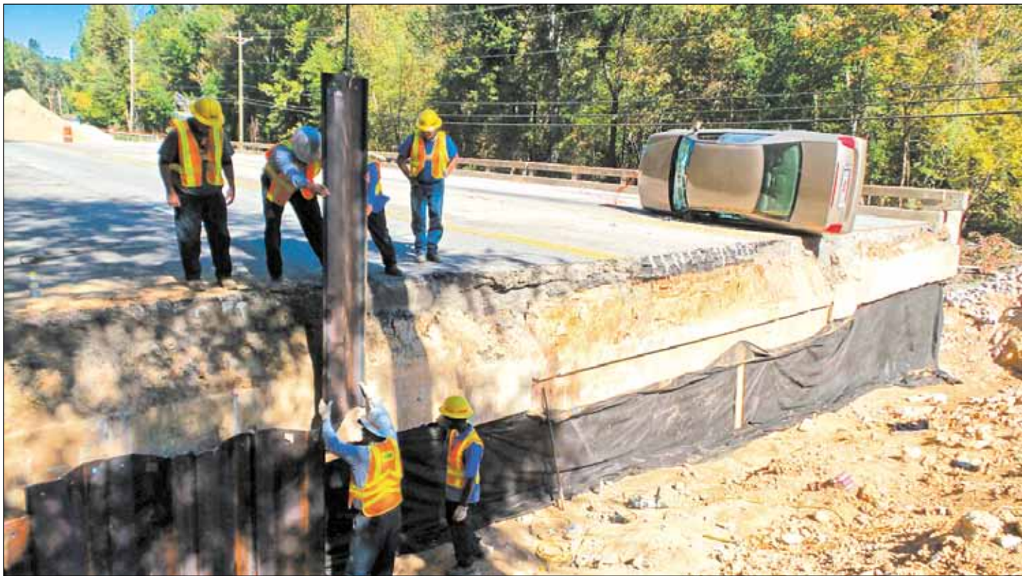
John Taylor of Aiken Maintenance guides a sheet piling into place with the help of his team doing work on the washed-out bridge headwall on Fairfield Road in Richland County. The work is part of SCDOT's ongoing flooding repairs across the state.
