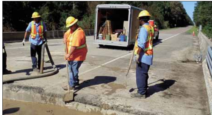
The Charleston Specialized Bridge crew repairs the headwall on a bridge along S.C. 41 in Berkeley County.
