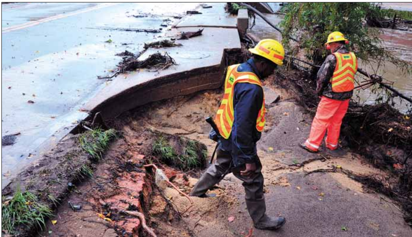
The District 1 Bridge inspection crew examines and monitors the washout of sidewalk around a bridge on U.S. 1 in Lexington on Oct. 5. SCDOT crews monitored bridges statewide during the flooding.
