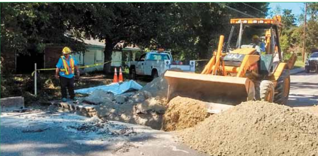
A crew uses a backhoe to fill a washed-out section of Lexington Avenue in Williamsburg County.
