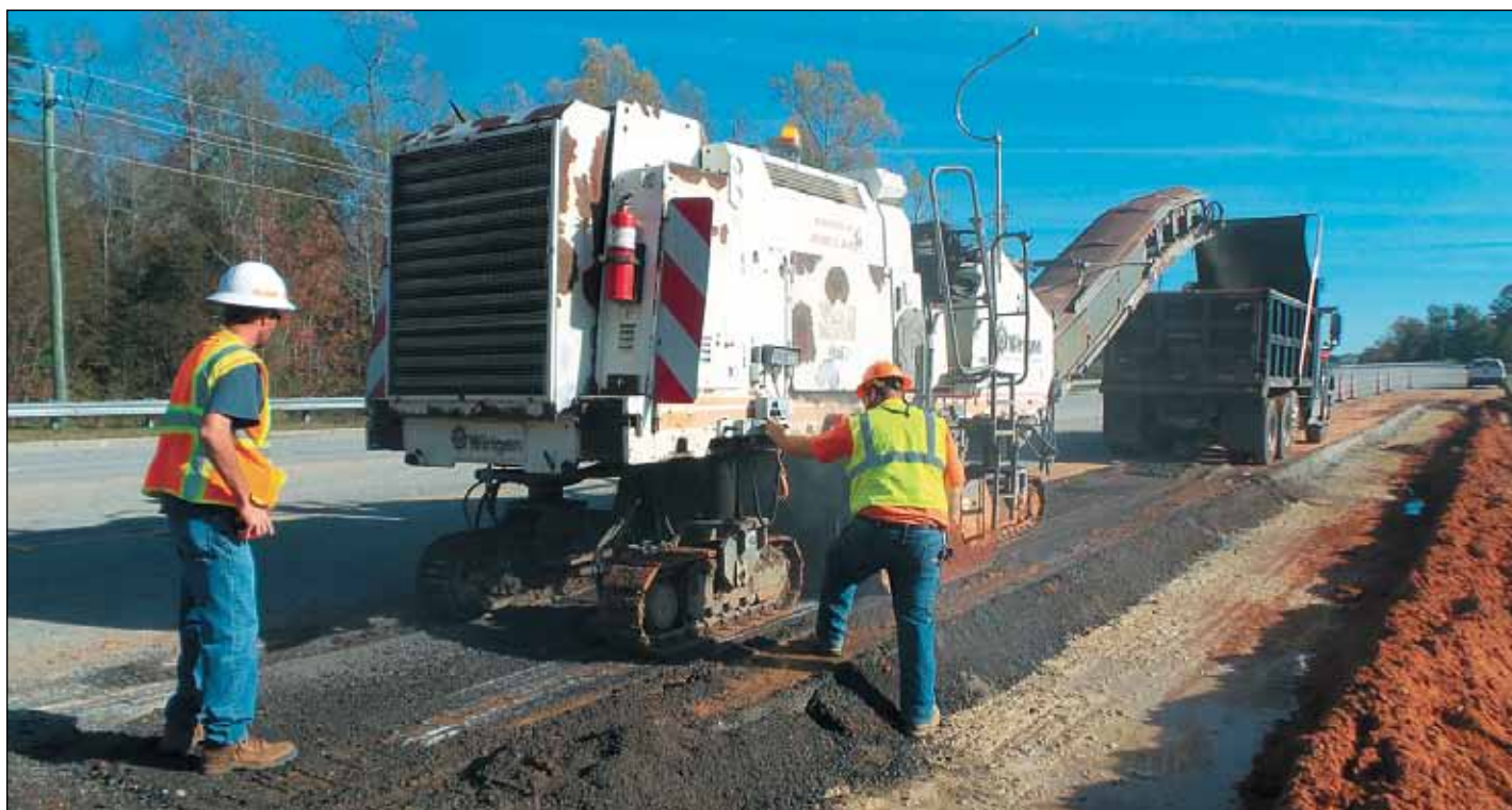
Allen Oxendine of SCDOT's Aiken Construction unit supervises the milling operation on U.S. 521 in Clarendon County on Nov. 20. The road was being prepared for paving to complete the repairs of a washed-out section of the road damaged by the October flooding.
