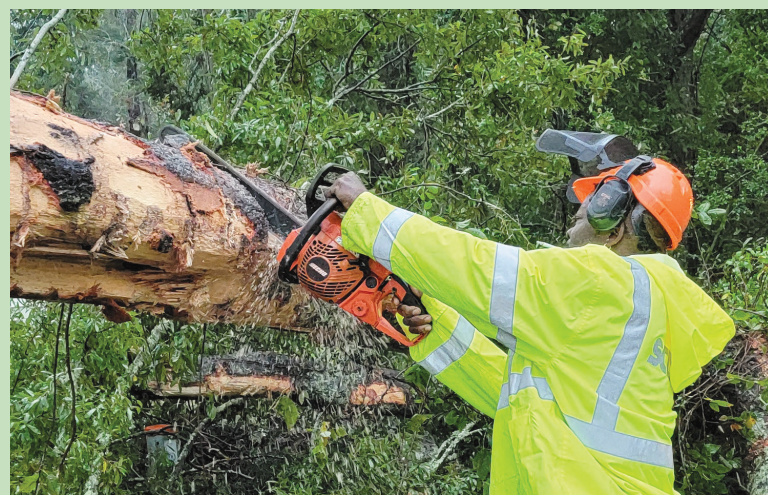
SCDOT crews used chainsaws to cut large trees that fell during the storm.
