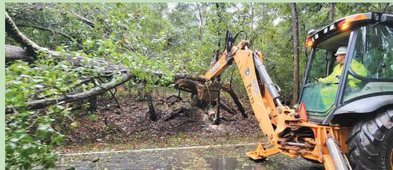
Backhoe operators lift and push trees and limbs to clear roadways immediately after Hurricane Ian passed by and through coastal areas.
