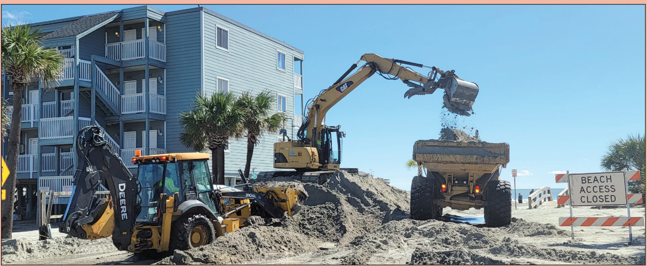
At Garden City, Horry County maintenance crews took the sand SCDOT removed from streets and placed it back on the beach to repair damage from the storm.
