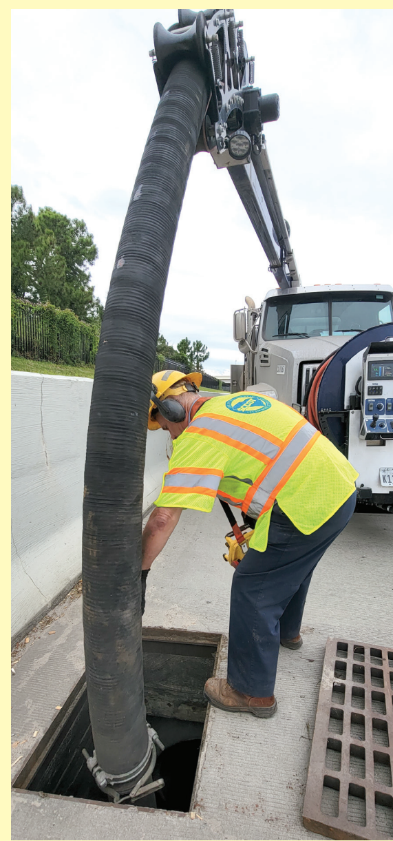
Drains are frequently vacuumed in flood-prone areas. Before the storm, extra drain cleaning was done to ensure drains could move water off roadways as quickly as possible.
