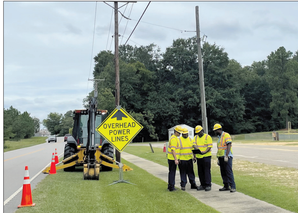
Foreman Ashton Walker reviews the Job Hazard Analysis form with Barnwell Maintenance employees Mike Jones, Zaviell Faust and Travis Grubbs.
