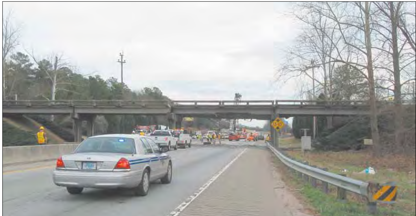
I-585 was closed for a day after a truck hit the California Avenue overpass and caused it to shift several feet. SCDOT crews worked through the night to demolish the damaged span by rush hour the next day. See more photos on page 26.
