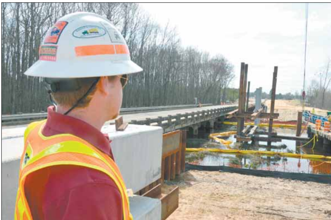
Robert Griffin of Florence Bridge Construction supervises the drilling of bridge pilings over Lake Swamp as part of the widening project of U.S. 76 near Timmonsville. The project widens 3.75 miles of U.S. 76 and associated side roads to accommodate the new alignment.
