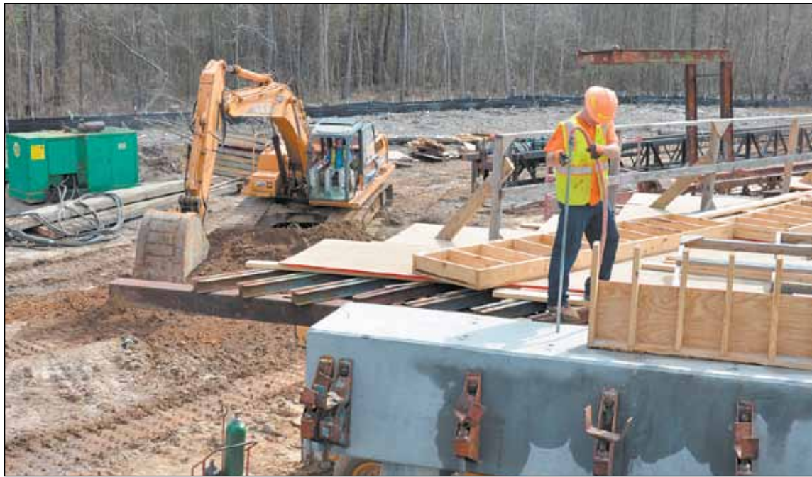
Contractors work on a bridge cap on the TV Road bridge over Black Creek.
