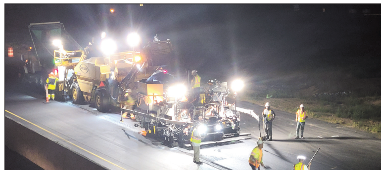
Five hundred thousand tons of asphalt was used on the project. Here, crews do paving overnight on I-85.
