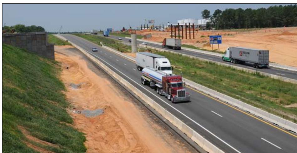
The I-520 and I-20 interchange will be the new exit 6 on I-20.
