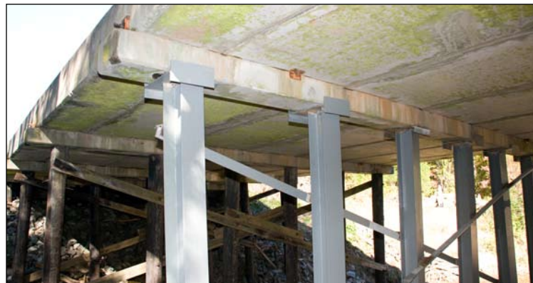
The Burris Road bridge over Turkey Creek was damaged by high water. District 4 employees repaired the bridge, replacing wooden pilings with steel pilings driven into the creek bed.
