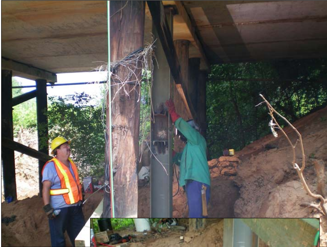
Chris Napoli and Craig Kyle replacing the support on Glenwood Road bridge.
