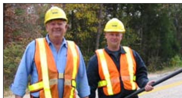
Right-of-way crew members Buck Taylor left, and Ricky Michau trim vegetation on SC route 97.
