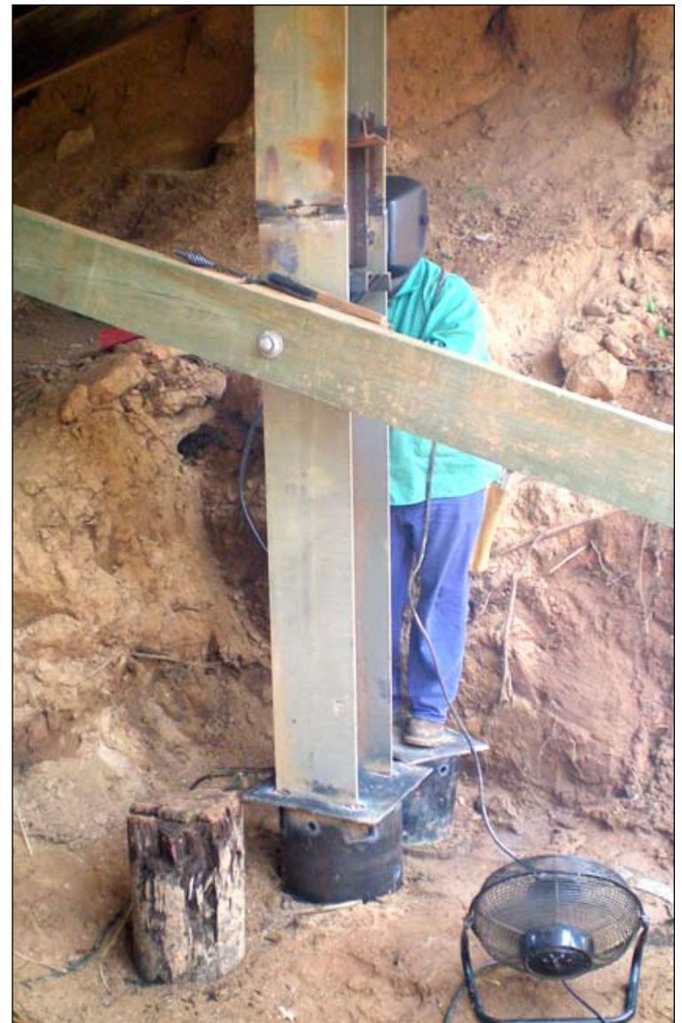
Pickens Maintenance employees are repairing support beams under the bridges. On the ground, the old wooden support has been cut away. Water rushing under it has caused erosion.
