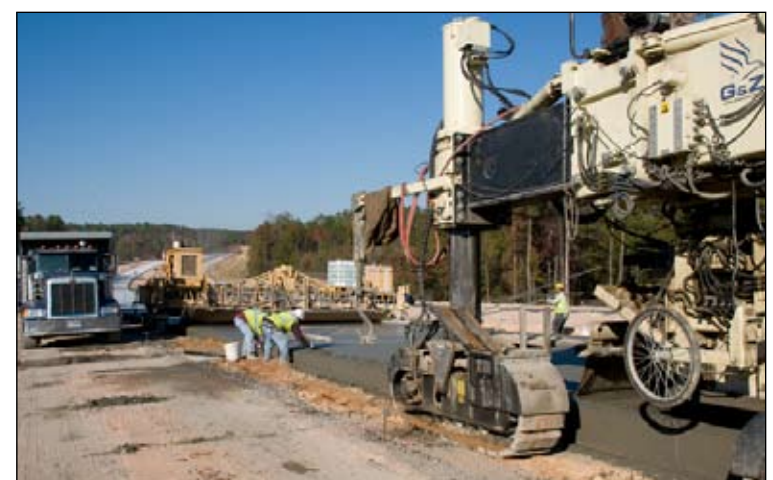
In November, concrete paving began on the project. Here, contractors pave a section of the highway using a series of machinery that pours, forms and smooths the wet concrete.
