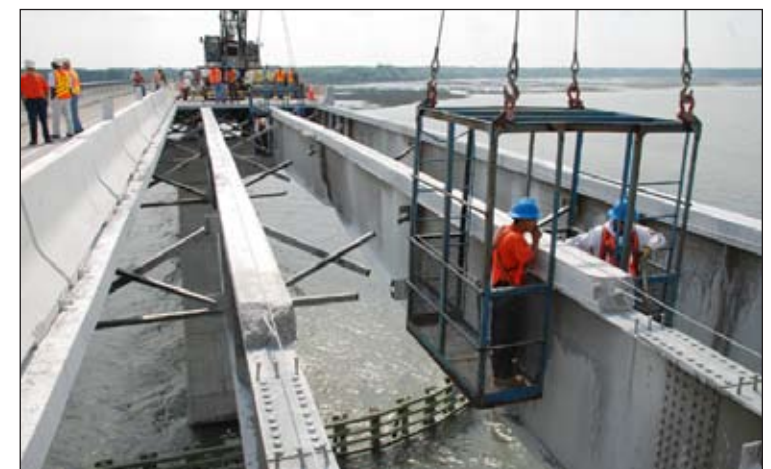
United Contractors employees are lowered by crane to cut existing framework from the damaged girders. Traffic on the bridge was limited to one lane during morning and afternoon rush hours.
