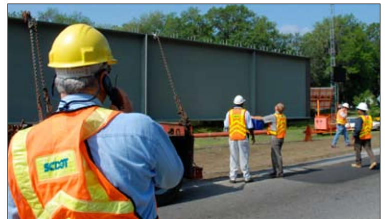
Clark watches as District 6 employees examine the first replacement girder to arrive from Augusta where it was manufactured. The 16,466-pound, 85-foot girder was delivered to the site with a police escort and cheering Beaufort motorists.
