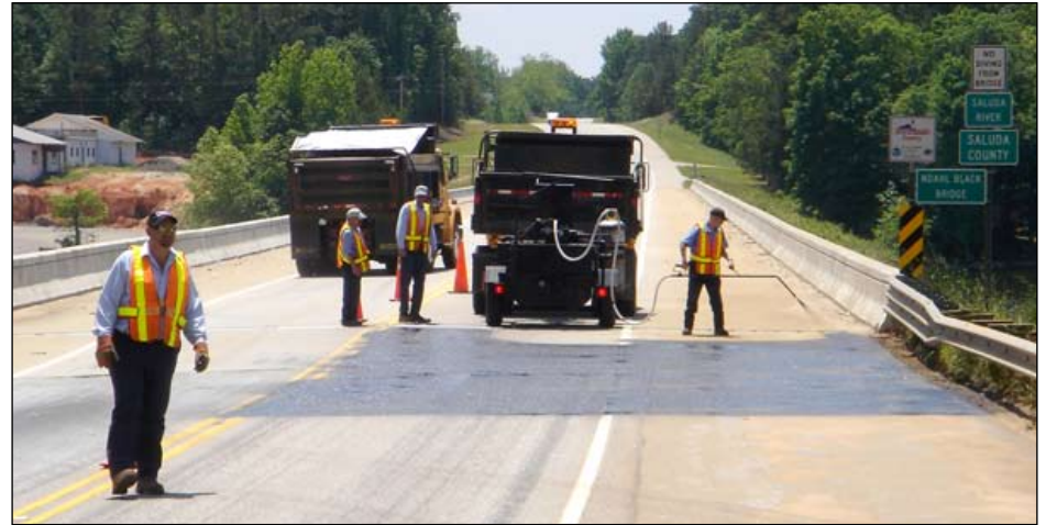
Johnny Lindler, Mike Lindler, Earl Smith, and Jeff Livingston prepare the road surface for a patch at Black's Bridge on the Newberry - Saluda county line.
