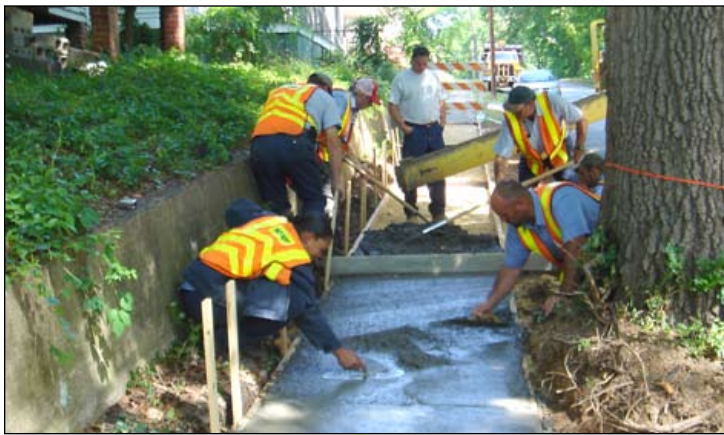
While the truck driver looks on, Newberry Multipurpose crew installs a long section of sidewalk in Whitmire. Pictured are (clockwise from left) Tina Laymon, Robert Icard, Leonard "Plug" Brown, truck driver, Ricky Smith, Jamie Glymph, and Hugh Pitts.
