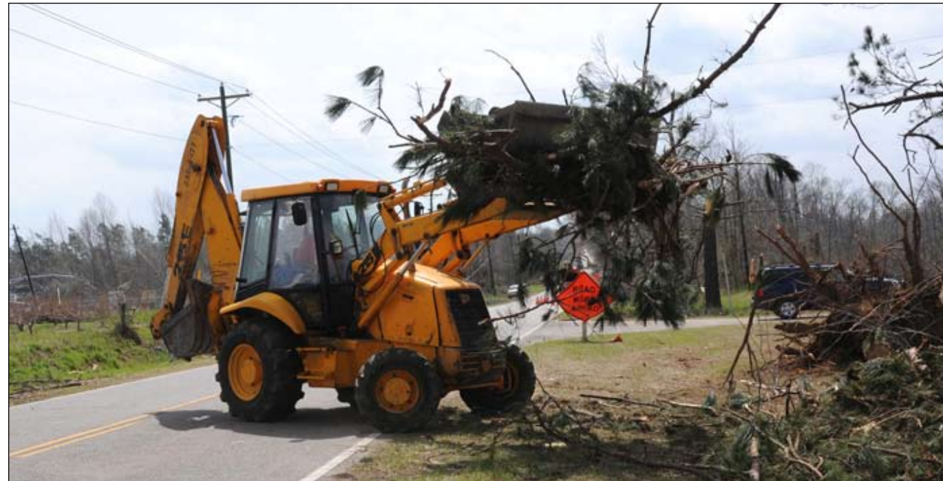
SCDOT employees clear debris from US 278 in Allendale County. Maintenance workers from Allendale, Barnwell, Orangeburg, Bamberg, Hampton, Colleton, Dorchester and Jasper counties were mobilized immediately after the storm to help clear the roads in Allendale County.
