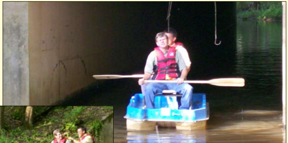
Mark DeZurik and Lee Neighbors inspect a culvert on I-385 Warrior Creek in Laurens Co. for possible rehab to the existing culvert. The inspection is part of the Interstate Rehabilitation Project for a section of I-385.
