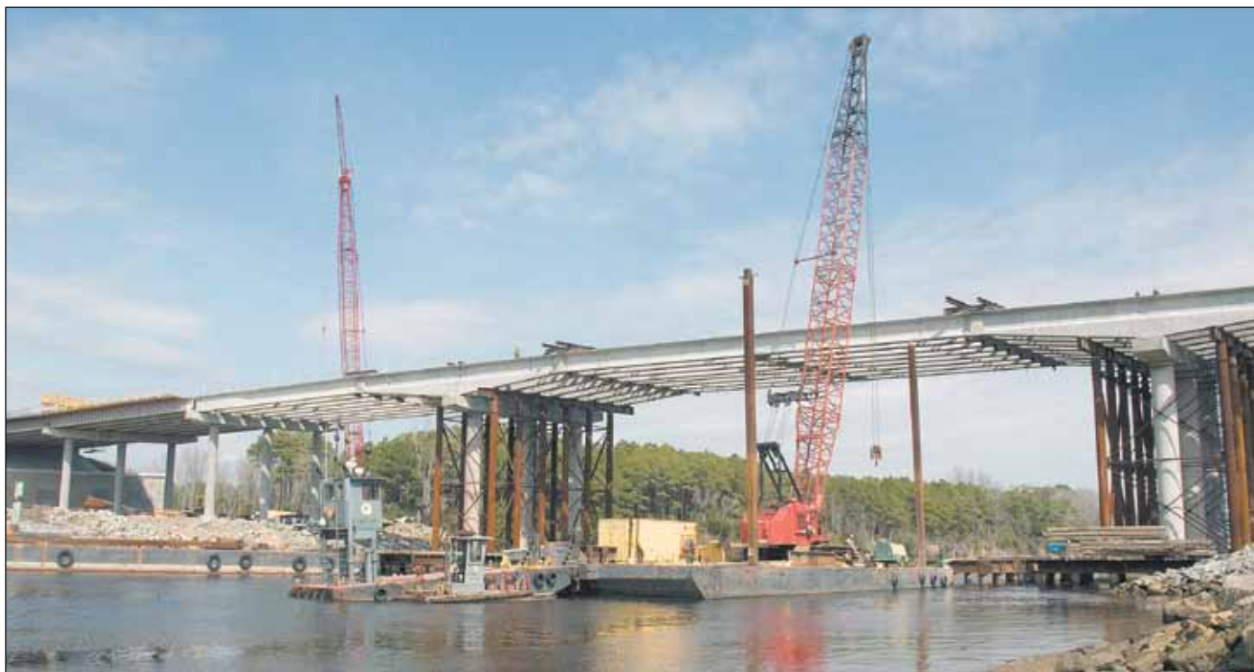
ABOVE: The North Myrtle Beach Connector bridge over the Intracoastal Waterway will connect North Myrtle Beach to the Carolina Bays Parkway.
