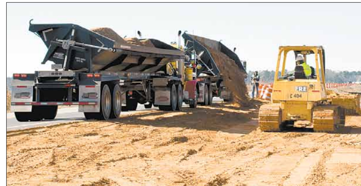
Side dump trucks are able to drop loads of dirt directly from the shoulder of the road. This prevents 'mud waves' in the marsh caused when heavy equipment travels on softer soil near the marsh.
