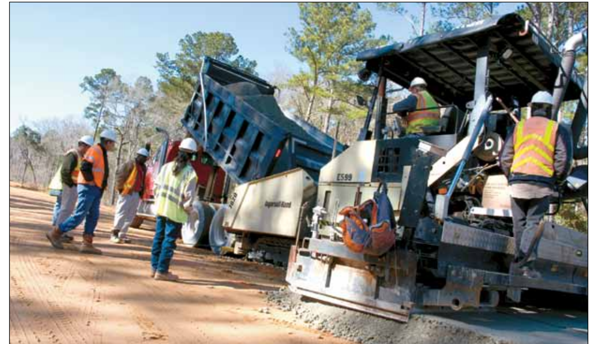
Away from the quiet zone, construction workers pave the concrete base layer of roadway using a high-density paver.
