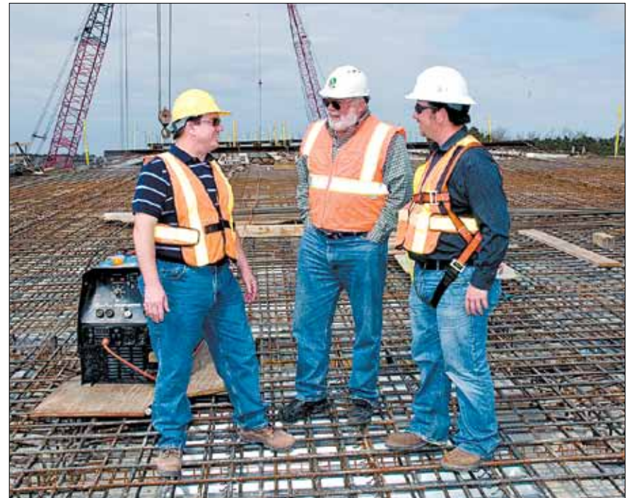
ABOVE: From left, Ken Hayes of Marion Construction, Bob Mobley of Wilbur Smith and Chris Cannon of Marion Construction discuss the project's progress.
