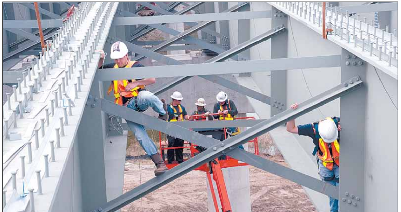
Joseph Cooper, left, and James Hammond, right, of Horry Construction check the cross frames and bolts on the Fantasy Harbor Bridge.
