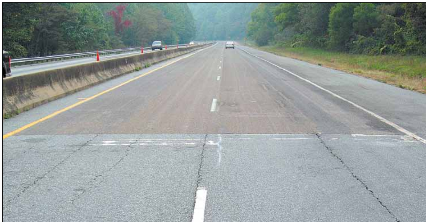
A high-friction asphalt resurfacing has been done along US 25 in Greenville County. Above, the contrast between regular pavement and the high-friction asphalt can be seen at the starting point of the resurfacing project.
