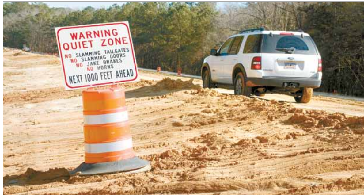
Construction workers near the area are required to keep the work zone area quiet due to the nesting eagles.
