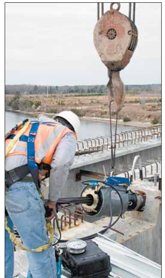
RIGHT: Willie Whipple of Freyssinet pulls cables that run through the girders of the bridge.
