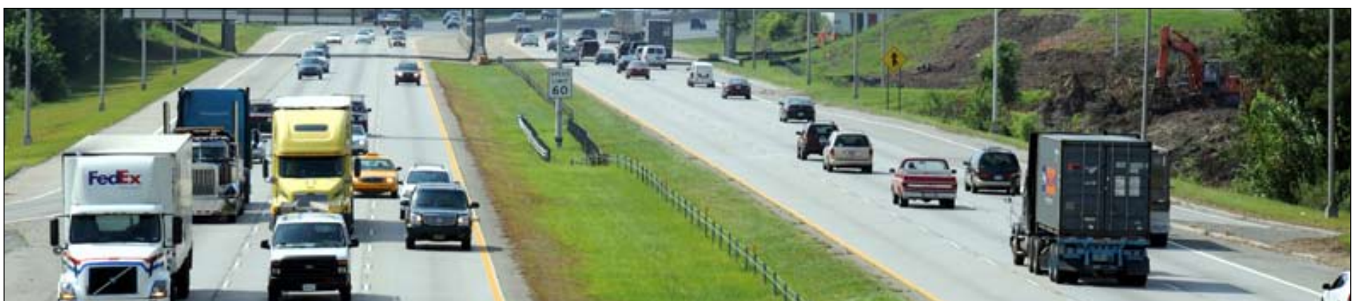
Clearing has begun for the widening of Interstate 26 in Charleston between Ashley Phosphate and Interstate 526.
