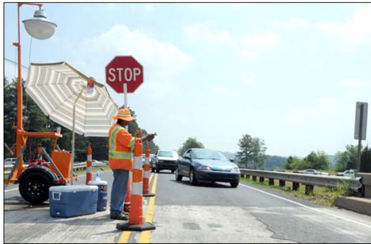
Juan Swope of Protection Services works traffic control around the Landrum Bridge repair work in Spartanburg County. Traffic control was done 24 hours a day while the repairs were made to the bridge.
