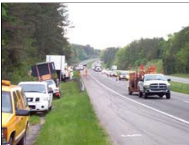
PHOTOGRAPHS BY DOYLE WAITES/NEWBERRY CONSTRUCTION Newberry Construction prepares a work zone for nighttime interstate work.
