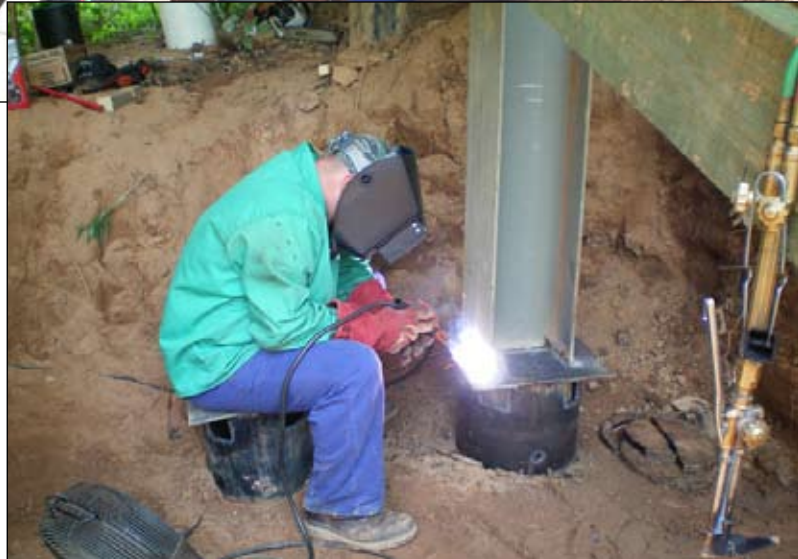
Craig Kyle, of Pickens Maintenance, is welding a new I-beam support under the bridge at SC 135 and Glenwood Road.
