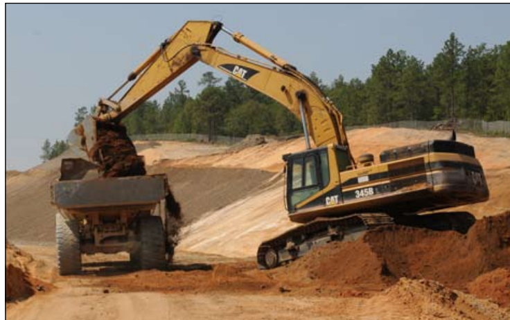
PHOTOGRAPHS BY ROB THOMPSON/THE CONNECTOR Dump trucks haul 27 cubic yards of fill with every trip. Large quantities of fill is required due to the changes in elevation along the roadway.
