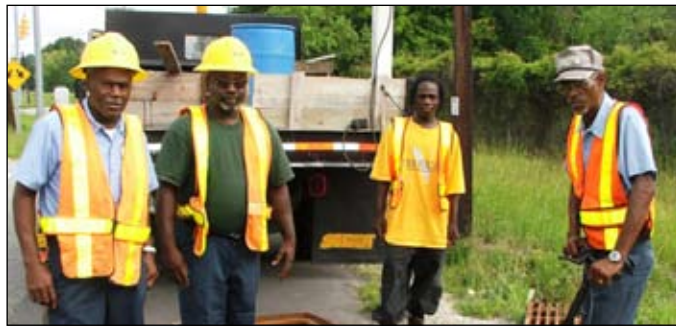
The driveway/concrete crew is: Leon Adams, John Gethers, Dennis Maxwell and Kenneth Bradley.
