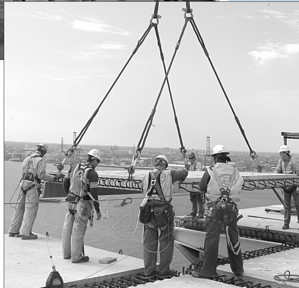
LEFT: Crew members place the last piece of the bridge deck in place.
