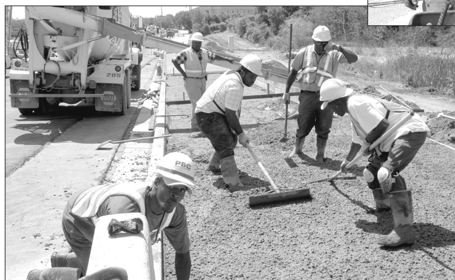
Workers pour the sidewalk for the bicycle and pedestrian lane on the Mount Pleasant side of the bridge.
