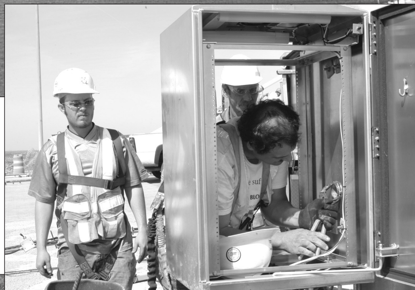
Workers prepare to an electrical box as part of the bridge's intelligent transportation system.
