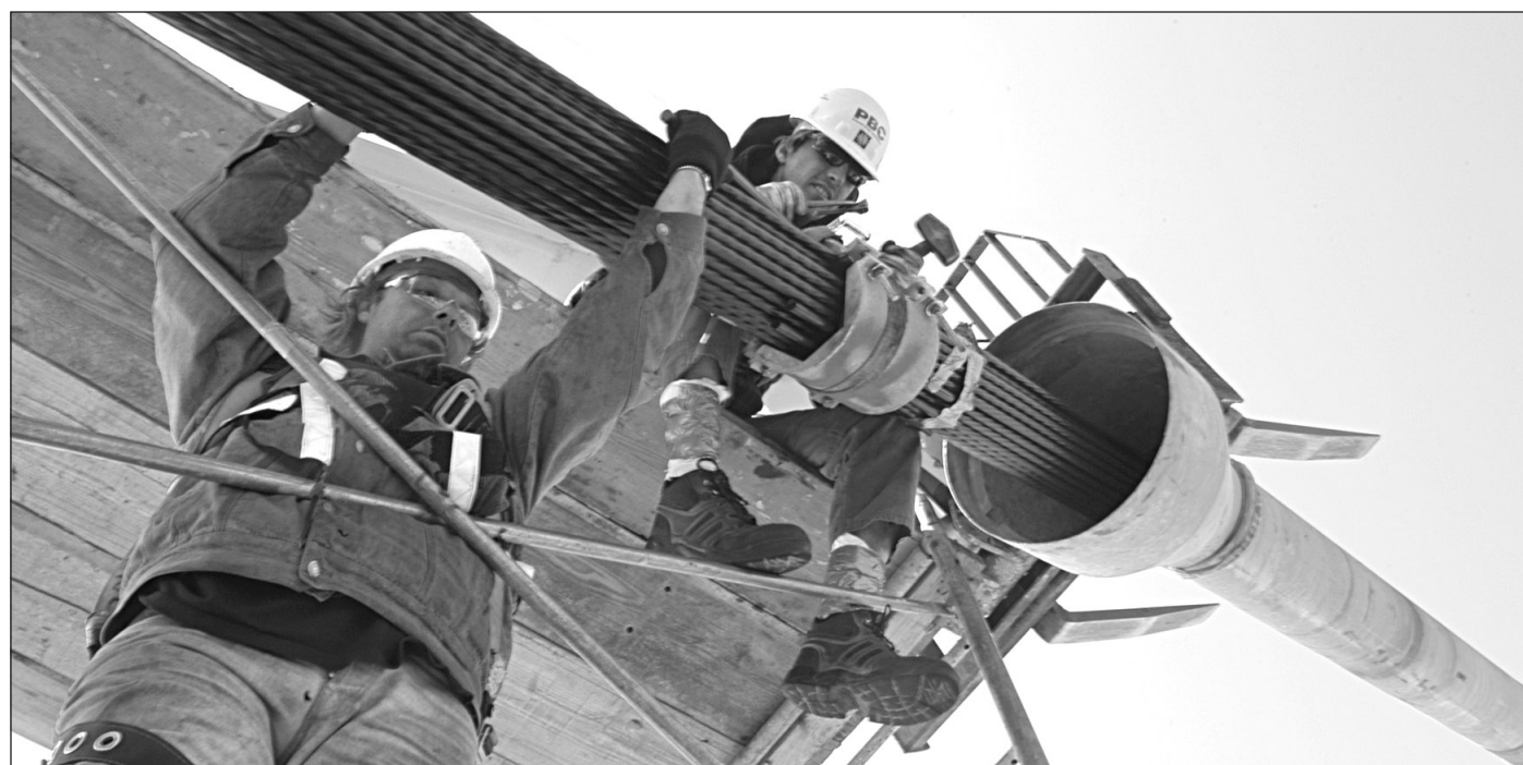
Bridge workers put the finishing touches on one of the strands of cable.
