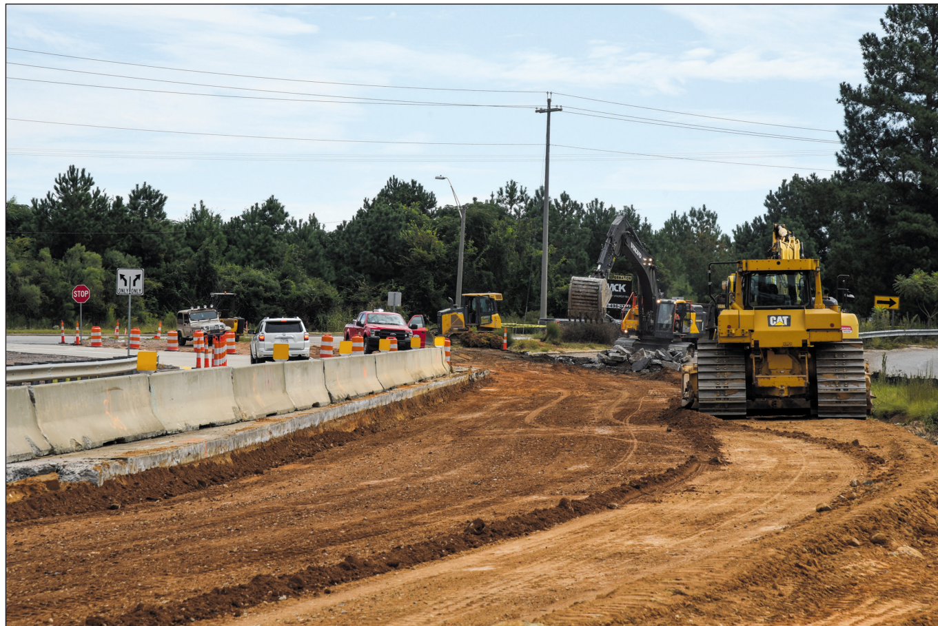
Work is ongoing at I-20 at Martintown Rd. (Exit 1) in Aiken County on Sept. 24, 2020.
