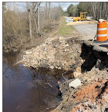
BEFORE: The failure is shown here on Spencer Road in Sumter County.
