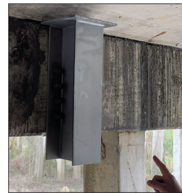
A further insurance to the slab-pinning, the opposite end of the "walking slab" has saddles epoxy-anchored to support any additional movement that should not occur after the repair is completed.
