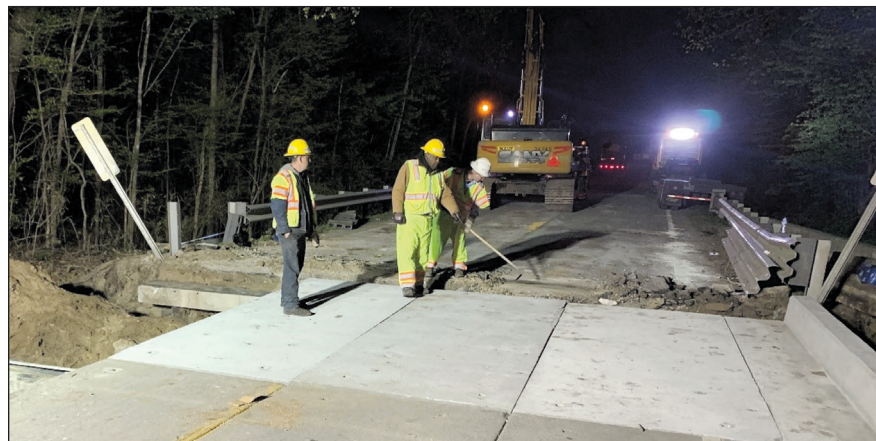
The work was done overnight on a Friday to be open early the next morning.
