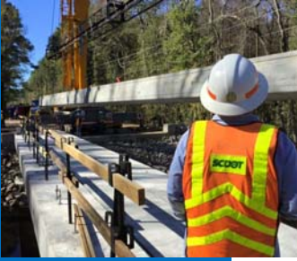
An SCDOT Bridge Crew sets precast bridge slabs on Lower Richland Boulevard. This new bridge was opened to traffic on November 24, 2015
