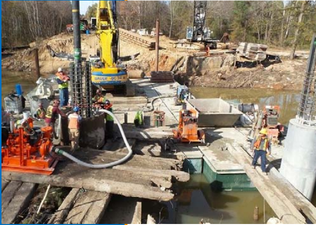
An SCDOT Bridge contractor is working to replace the US 176 bridge over Cannon's Creek in Newberry County. This bridge is scheduled to open by March 29, 2016.
