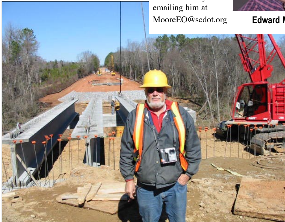
Floyd Long of Chester Construction inspects concrete beam placement on bridge project over Fishing Creek in Chester County.
