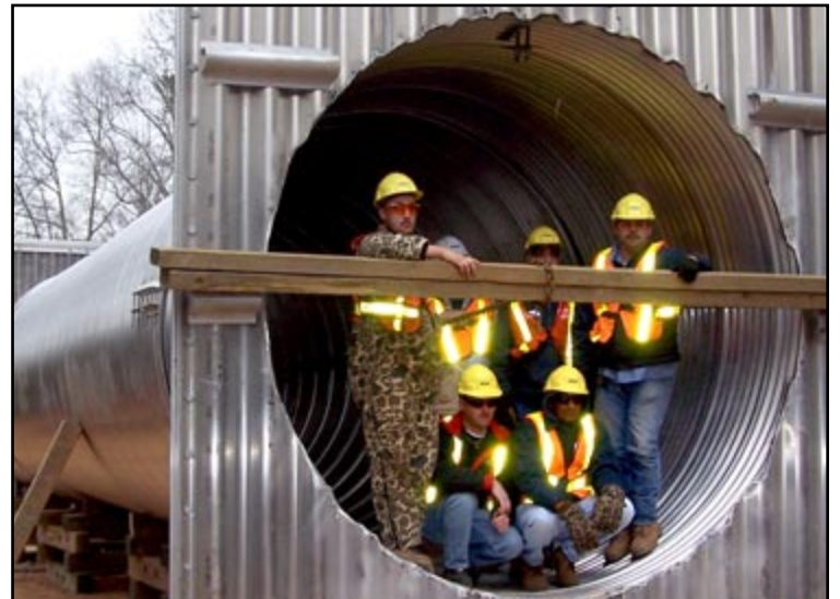
Just 24 hours before a winter weather threat hit the upstate, this crew was working hard to repair a road. On Jan. 28, James Charping, Brad Merritt, Trey Schmuck, Billy Frankmun, Earl Thompson, and Douglas Montgomery were waiting for a crane to arrive on McDuffie Street (S-04-149). A 12'5" wall holding a 50 foot, 108" aluminum pipe was set to be placed by the end of the day. After this, they were preparing for the snow and ice forecast to hit Anderson, SC.
