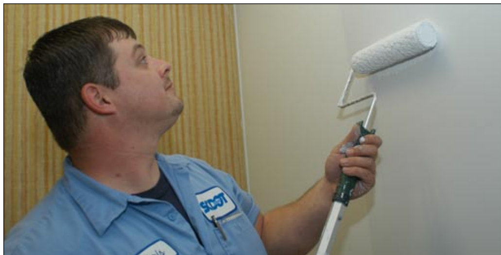
BELOW: Chris Huepenbecker of Building Maintenance applies a fresh coat of paint to a first floor office wall prior to Human Resources moving into the recently vacated space.
