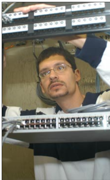
ABOVE: Greg Szymanski of IT Services reroutes network cables as part of the office moves at SCDOT Headquarters.
