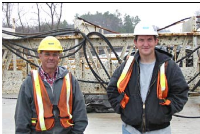
Eddie Mitchell, left, and Jason Wyatt inspect concrete deck pour on bridge replacement project on S.C. 49 in York County.
